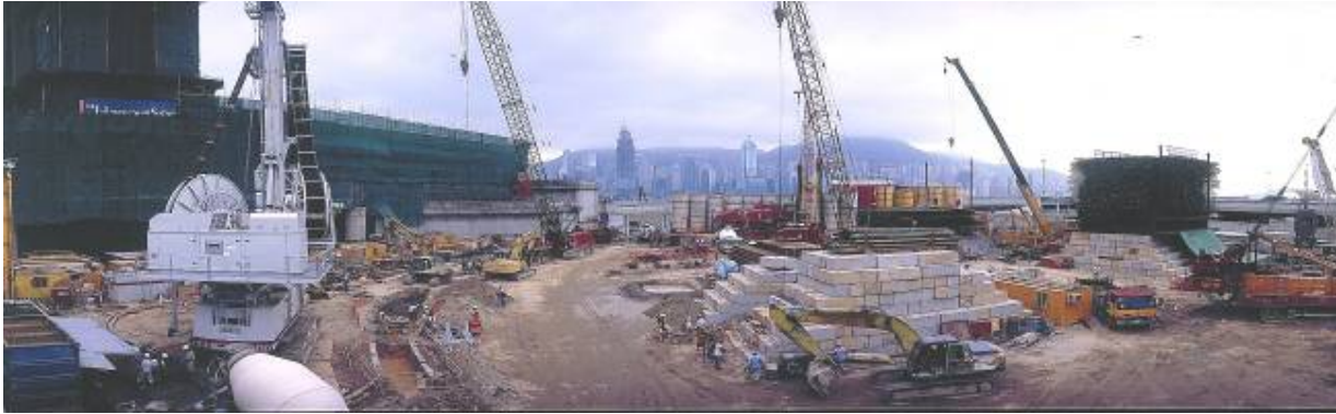
The site is located within the West Kowloon reclamation nearby the existing MTRC Kowloon Station.
