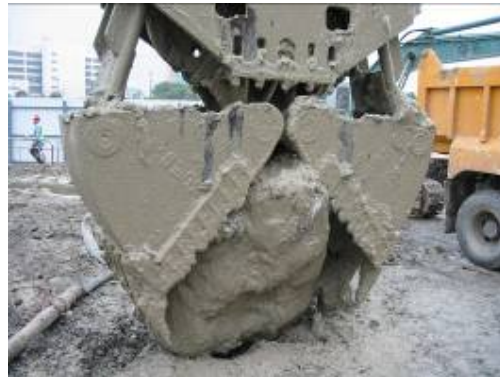
Presence of boulders was one of soil difficulties.
