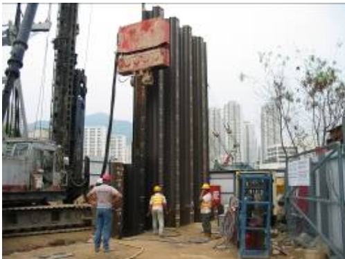
Driving sheet piles using high frequency vibration in order to minimize the effect of vibration on adjacent structures.
